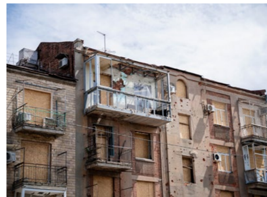
A common sight in many streets of Kharkiv: Entire rows of houses peppered with holes from missiles.
